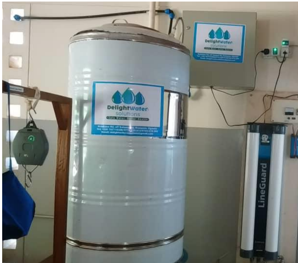
UV system in a Premium Cage installed with 750l smart tank at Gombe Hospital, Butambala financed by Islamic Centre for Education and Research.
